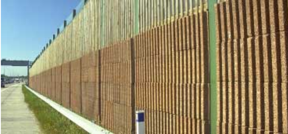
Noise Barrier Textural finishes and transparent materials may reduce the visual impact
