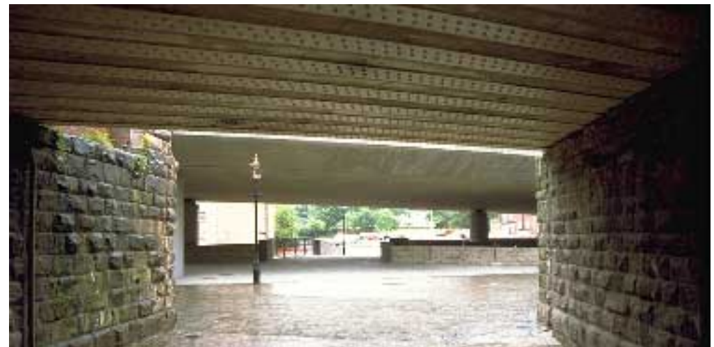
Bridge Underside Bats may roost under bridge decks and these should be inspected prior to maintenance operations
