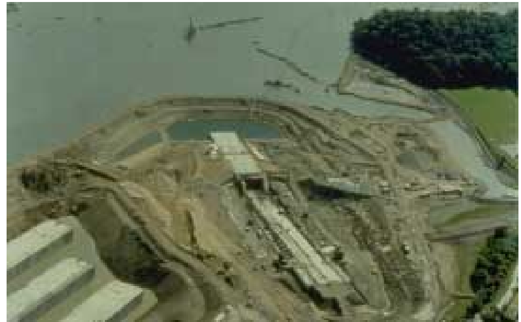
Conwy Tunnel Temporary works design and construction constrained by the need to protect the marine environment
