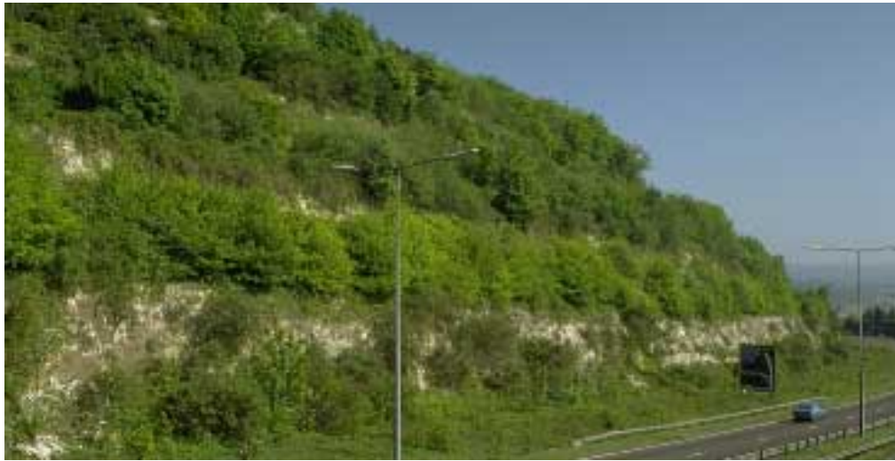
Rock Cutting Exposed geology adds interest, acts as a landmark, and over time may develop biodiversity interest
