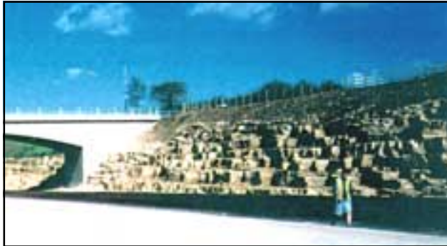
A417, Cirencester. The rock has been shaped to take advantage of its natural structure.
