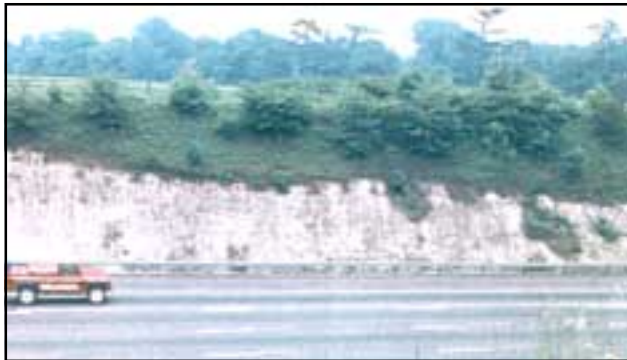
M25, Walton on the Hill. The chalk cutting has been formed with slope variation and small shelves.
