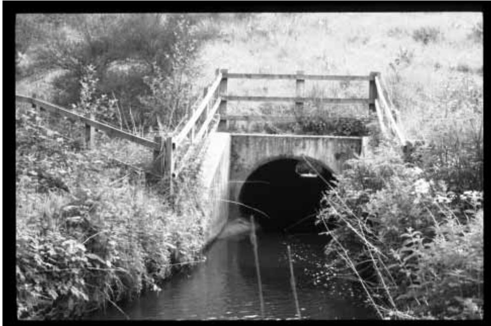
A 40 Haverfordwest, Wales. A typical cylindrical culvert. An underpass was installed nearby after the death of an otter on this stretch of road (figure 13).
