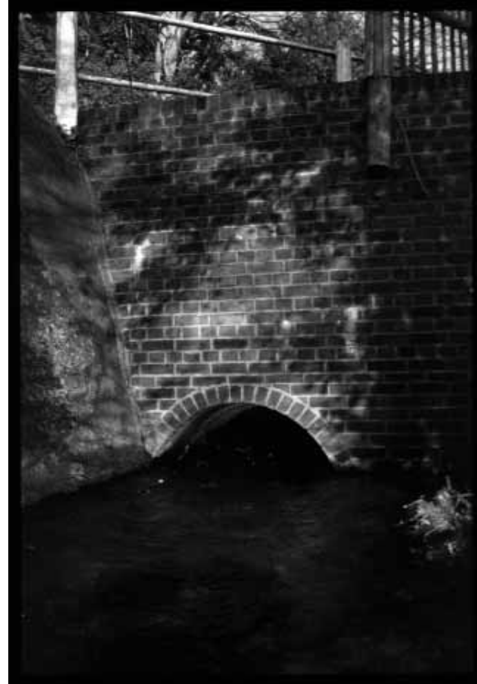
Another culvert, this time near Alresford, Hampshire, and the probable cause of death of two animals. An underpass has since been installed (figure 14).
