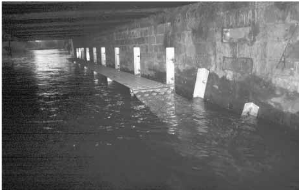
Bishopstoke, Hampshire. A ledge constructed of galvanised steel has been bolted on to this structure. (Environment Agency).
