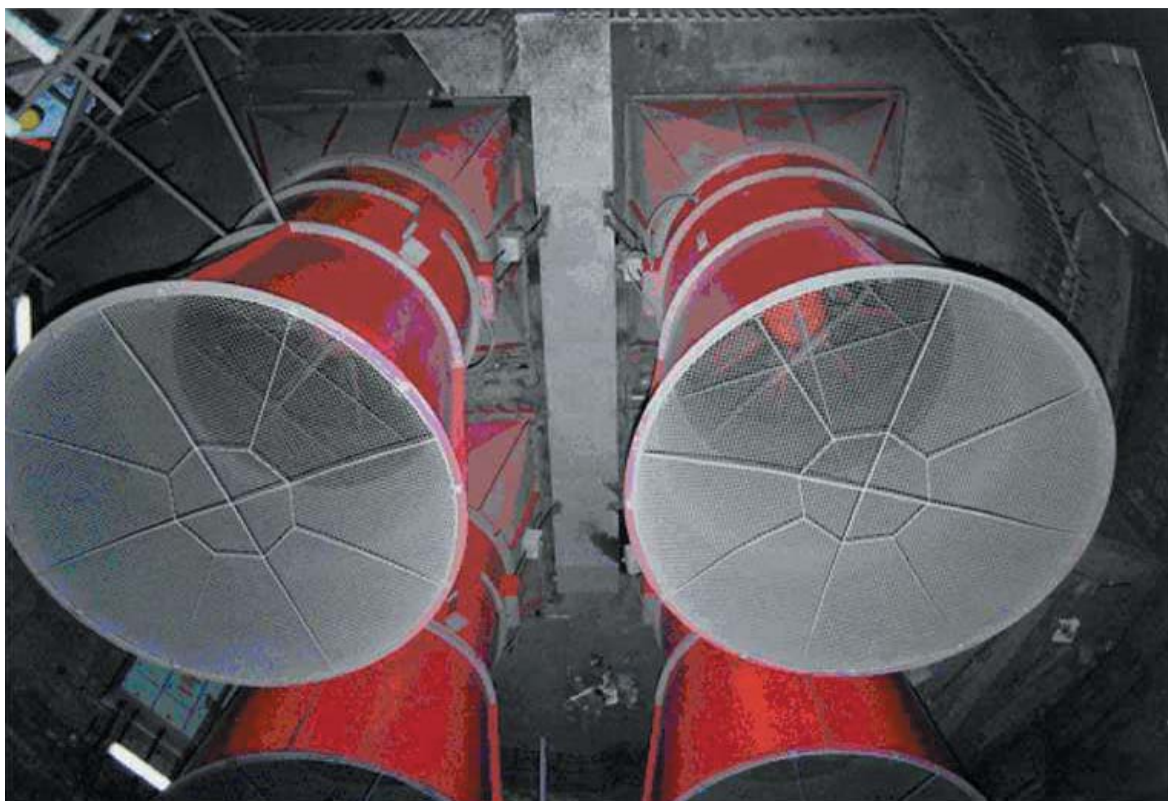
Figure 7.2: Fixed Axial Fans over Supply/Extract Shaft
