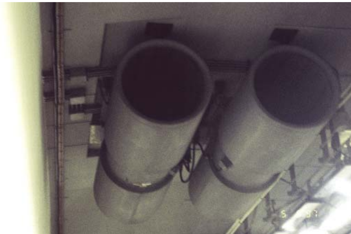
Figure 7.1: Jet Fans providing Longitudinal Ventilation
