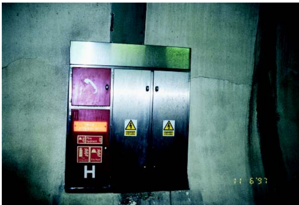
Figure 10.1: Tunnel Emergency Panel
