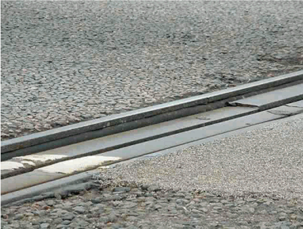
Fig 8: Viaduct (Insitu concrete deck) Built 1986 Damage to the West Deck Expansion Joint- Rail broken in the middle and level difference
