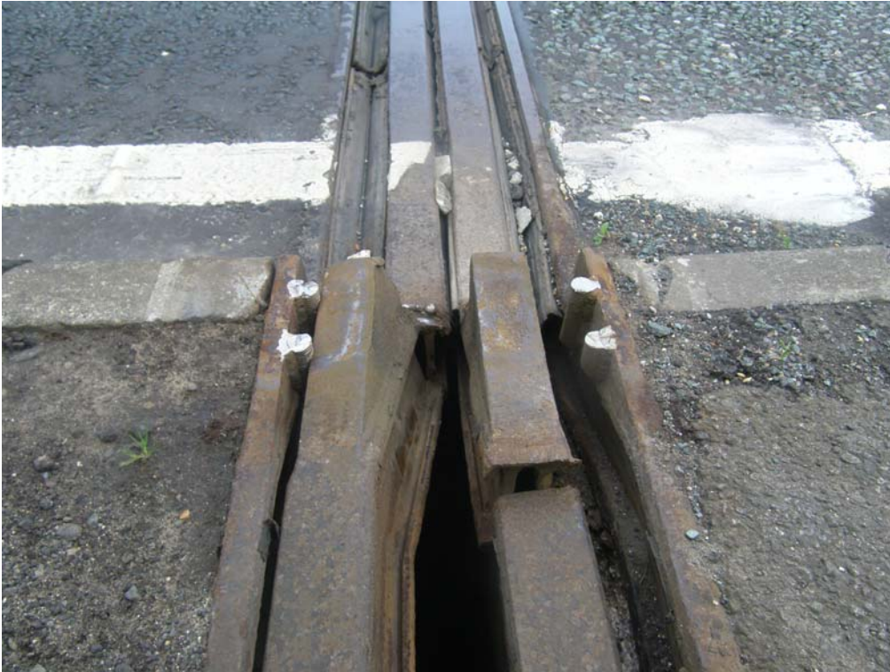
Fig 6 Cable Stayed Bridge (Composite steel-concrete deck) Built 1991 Trimmer Beam Support Steelwork corroded
