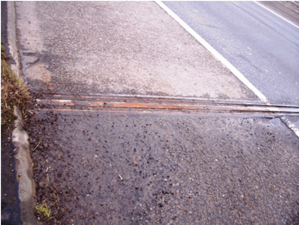
Fig 9: Viaduct (In-situ Prestressed Concrete) Built 1990 Corrosion to rails and debris in seals
