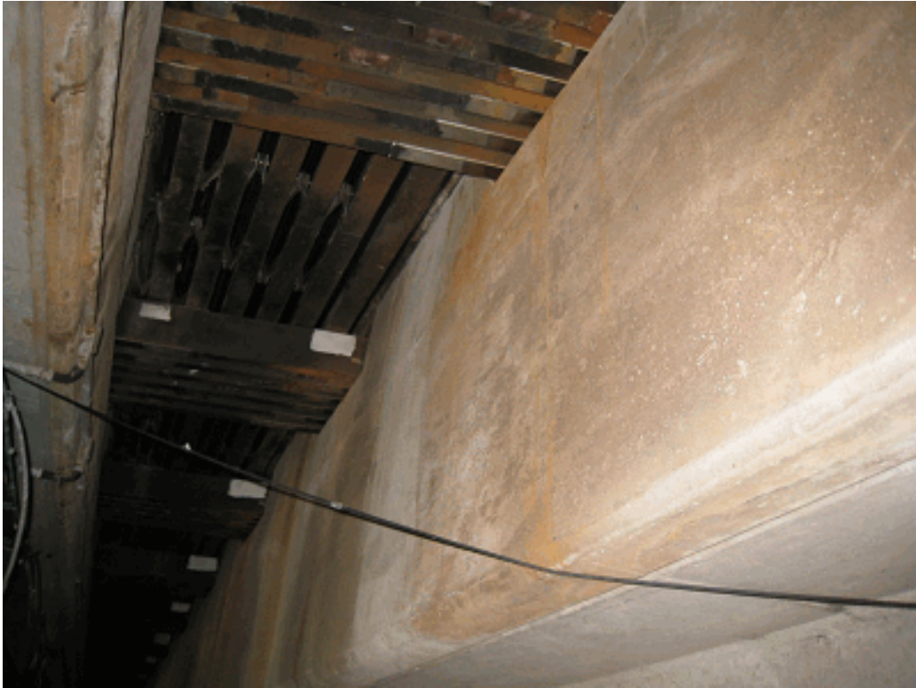
Fig 4: Cable Stayed Bridge (Composite steel-concrete deck) Built 1991 Rust staining from expansion joints over pier (Seal replacement stopped water ingress, circa 2007)
