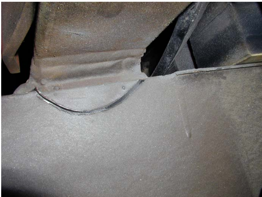
Fig. 3: Cable Stayed Bridge (Composite steel-concrete deck) Built 1991 Fracture in the support joist immediately below the welded connection to the rail
