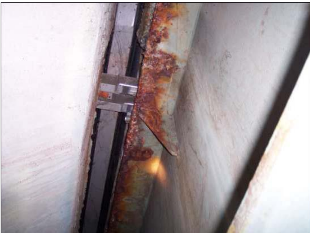
Fig 7: Viaduct (Precast Prestressed Concrete) Built 1976 Failure of joint on footway. Seal failed between rails on carriageway
