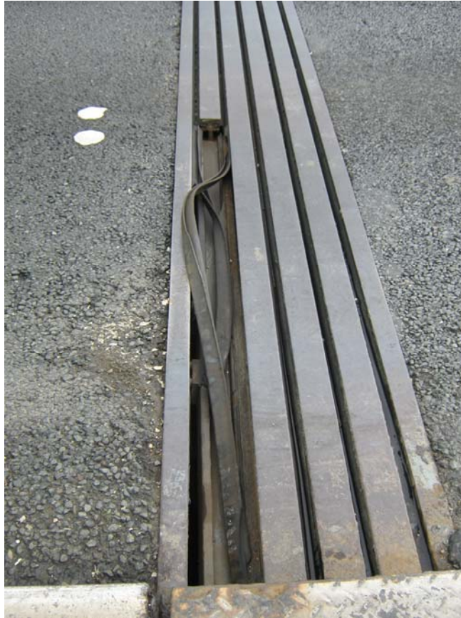
Fig 2: Viaduct (Precast Prestressed Concrete) built in 1993 The damaged rail has been taken out of the joint and corrosion is visible on the rails
