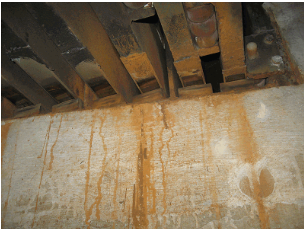
Fig 5: Cable Stayed Bridge (Composite steel-concrete deck) Built 1991 Corrosion to expansion joints sliding plates over pier, circa 2007
