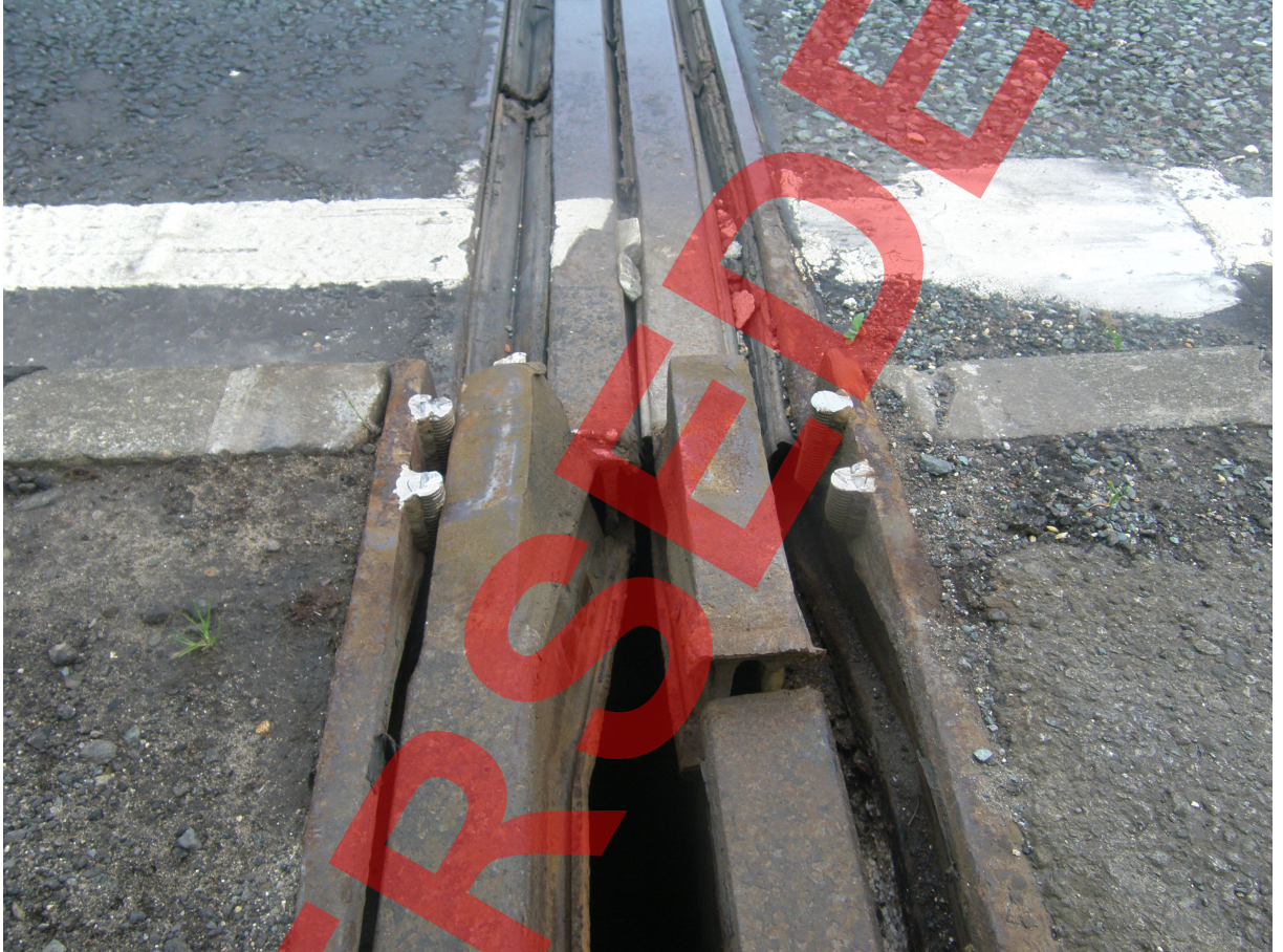
Figure E.6 Viaduct (Pre-cast pre-stressed concrete) Built 1976- Failure of joint footway. Seal failed between rails on carriageway
