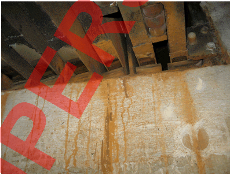
Figure E.5 Cable-stayed bridge (Composite steel-concrete deck) Built 1991 - Corrosion to expansion joint sliding plates over pier, circa 2007
