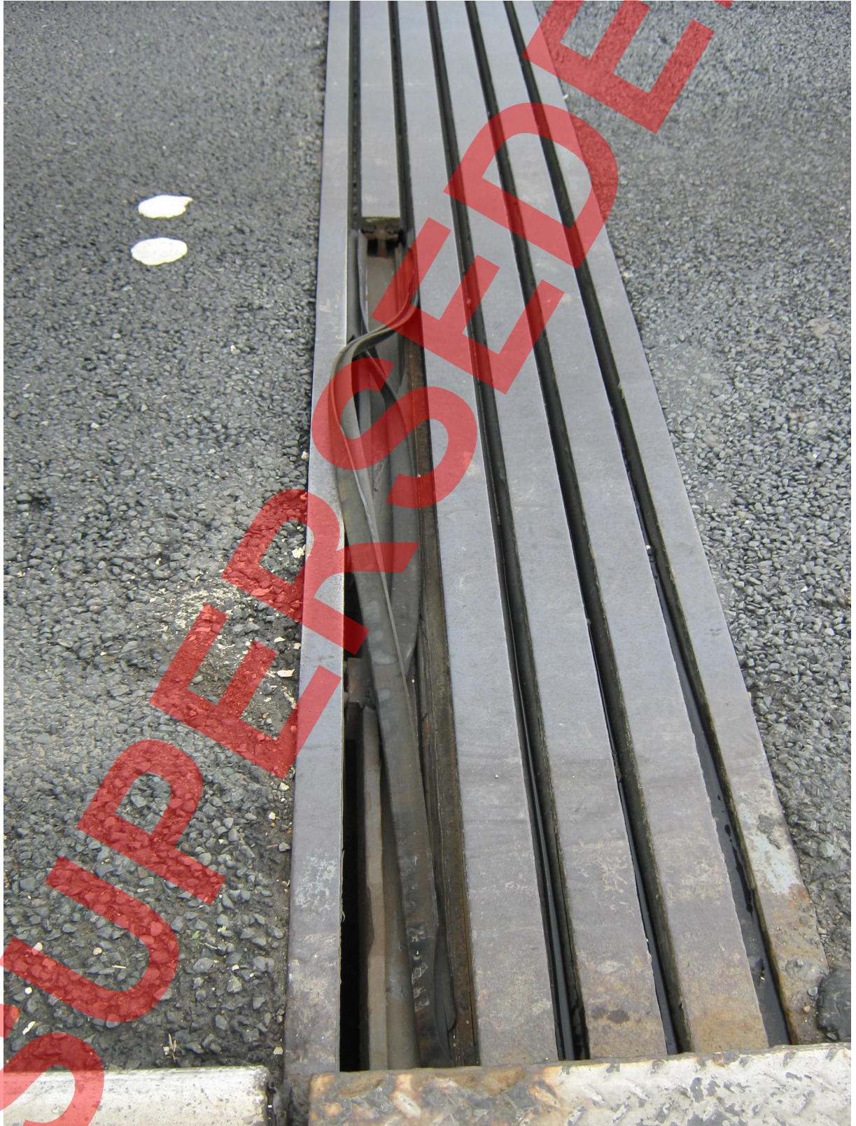
Figure E.2 Viaduct (precast prestressed concrete) built in 1993- The damaged rail has been taken out of the joint and corrosion is visible on the rails
