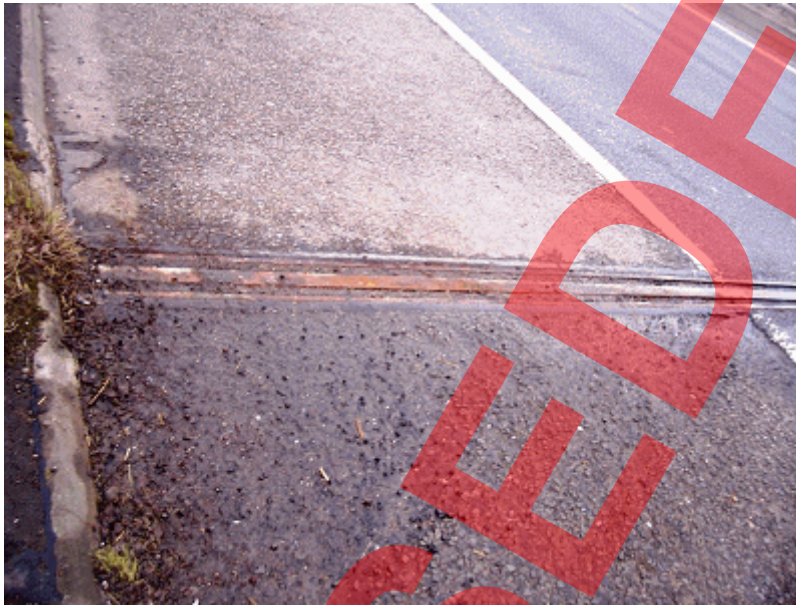
Figure E.9 Viaduct (in-situ pre-stressed concrete). Built 1990 - Corrosion to rails and debris in seals
