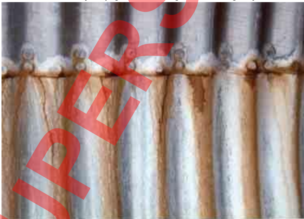
Figure B.8 Deterioration to side plates in a plain galvanised bolted segmental CSBS caused by seepage below the edge of the carriageway
