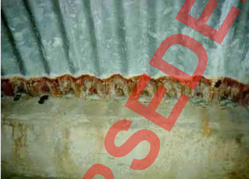
Figure B.9 Deterioration at the arch seating of a plain galvanised arch structure due to seepage and ponding of water containing de-icing salts
