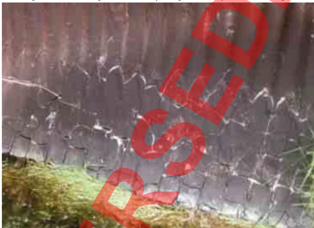
Figure B.5 Cracking in a bitumen paving due to exposure to sunlight
