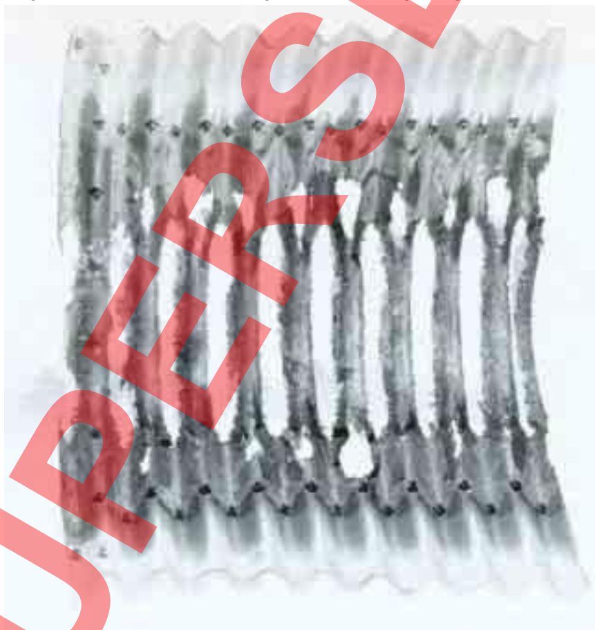
Figure B.1 Example of extreme corrosion in the invert of a structure subject to scour (this 30 year old structure was not provided with a paving or bitumen coating)
