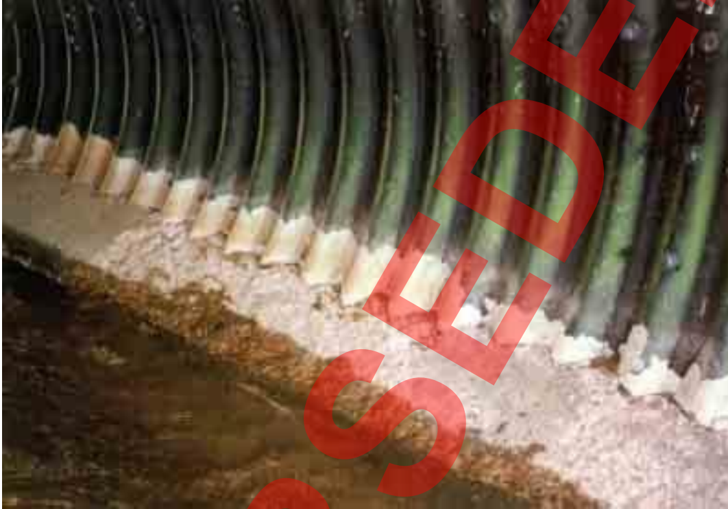
Figure B.11 Damaged bitumen coating caused by overtopping of paving during turbulent flow
