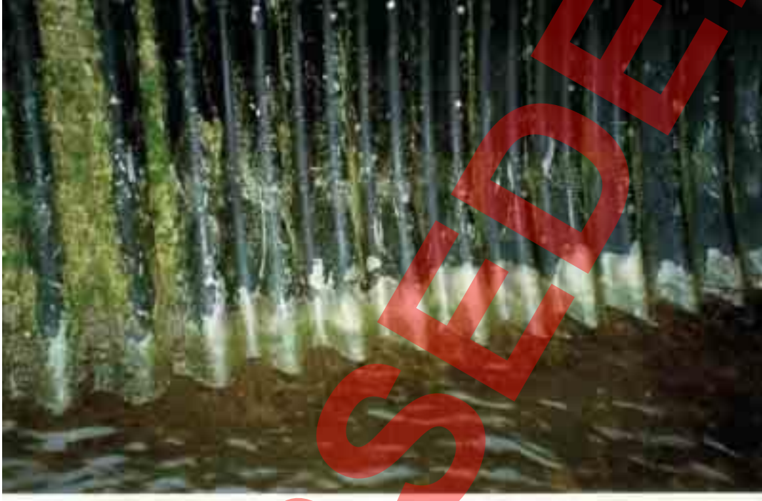
Figure B.3 Damaged bitumen coating caused by overtopping of paving during turbulent flow
