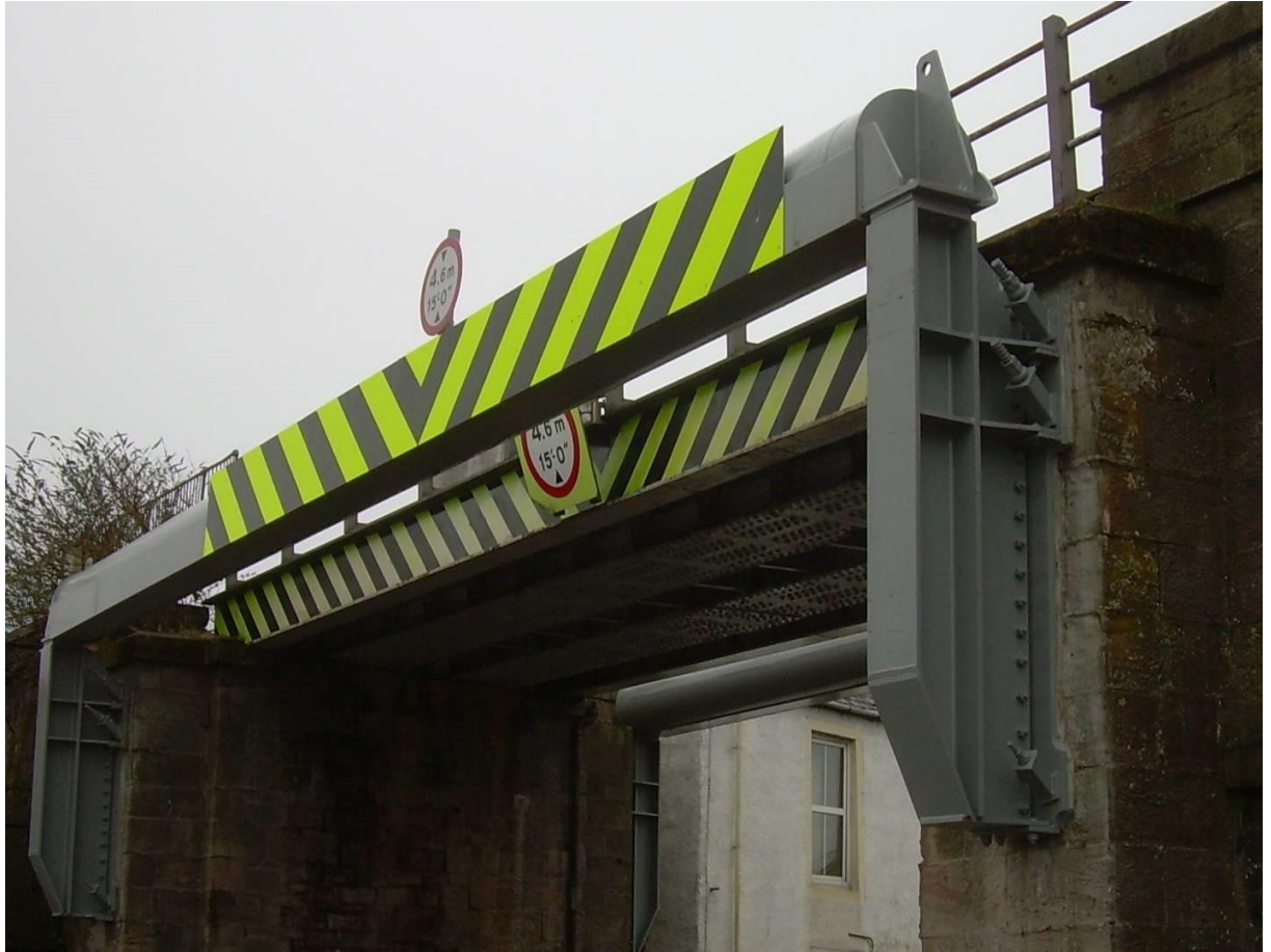
Figure A.3 Circular collision protection beam to flat soffit bridge showing abutment supports
