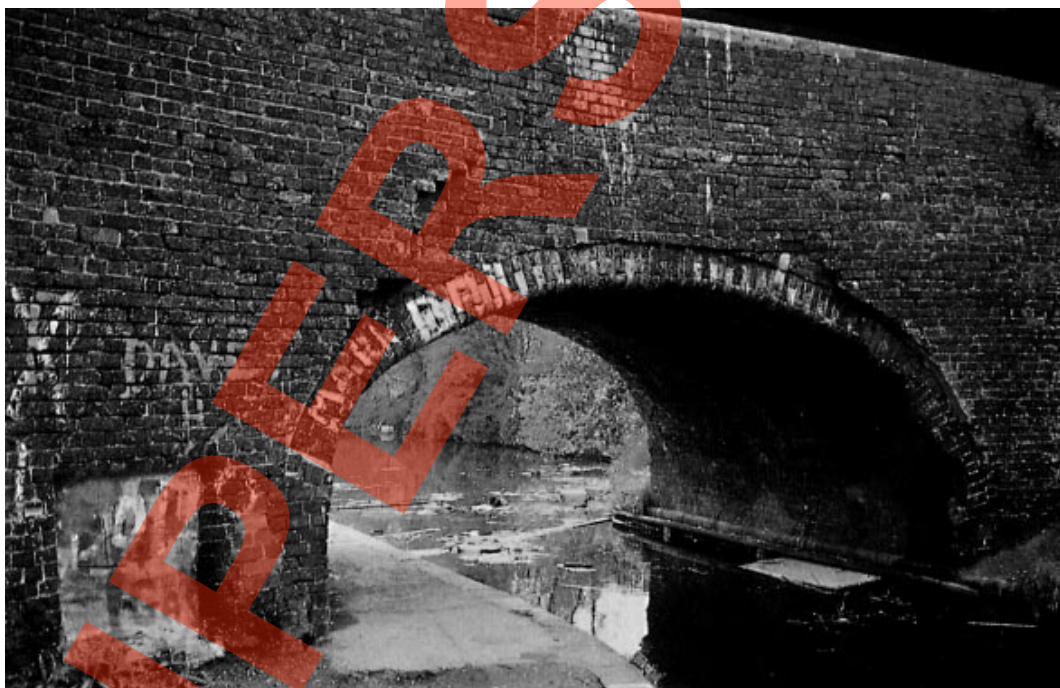
Plate 9 This illustrates the movement of spandrel walls.
