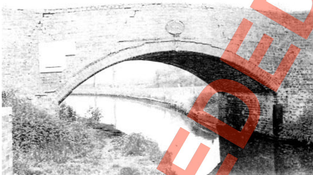
Plate 11 This shows cracking of the spandrel/parapet walls which suggest a flexible arch barrel.
