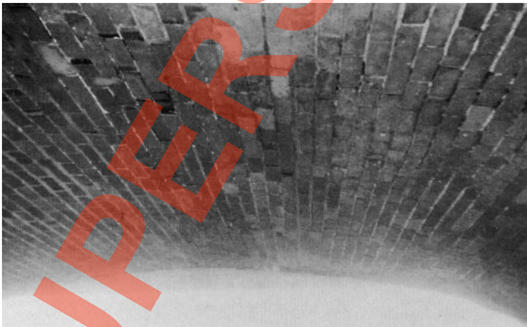
Plate 7 This shows a localised deformation of an arch which would perhaps reduce its Condition Factor by 0.1.
