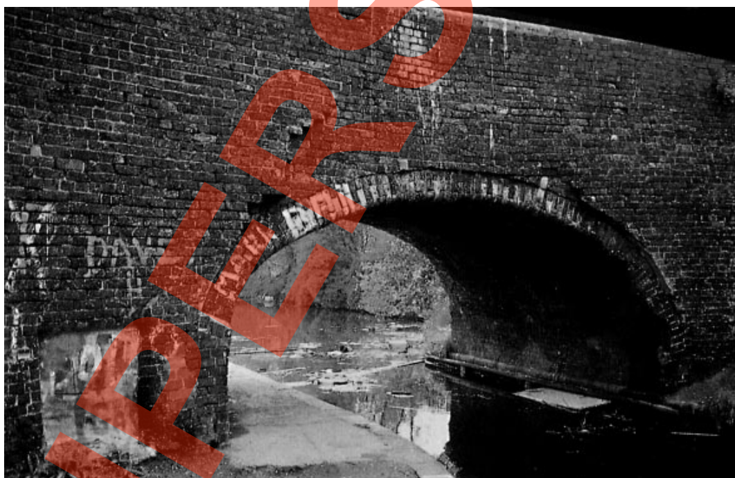
Plate 9 This illustrates the movement of spandrel walls.
