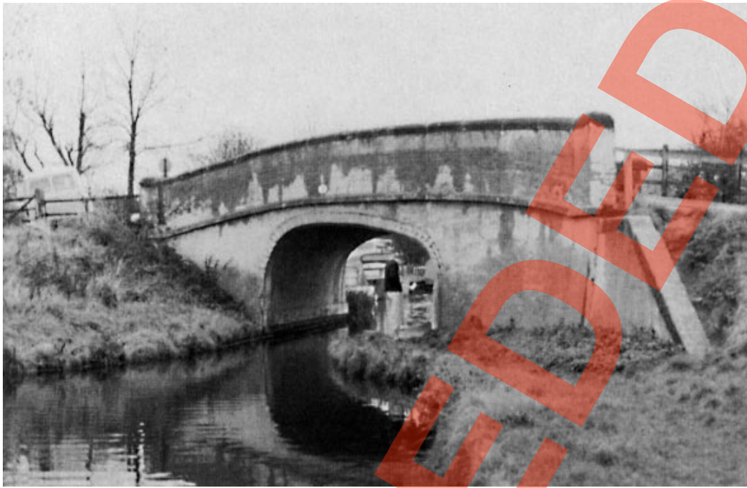
Plate 6 This shows an arch which has become grossly deformed and flattened in shape. The MEXE method would not be suitable for assessing its carrying capacity and instead it should be assessed from first principles.
