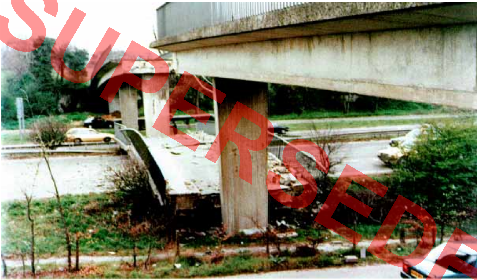
PLATE 2 COLLAPSE OF A DECK SPAN FOLLOWING A COLLISION FROM AN EXCAVATOR TRANSPORTED ON A LOW LOADER A2 PARK PALE ACCOMMODATION BRIDGE
