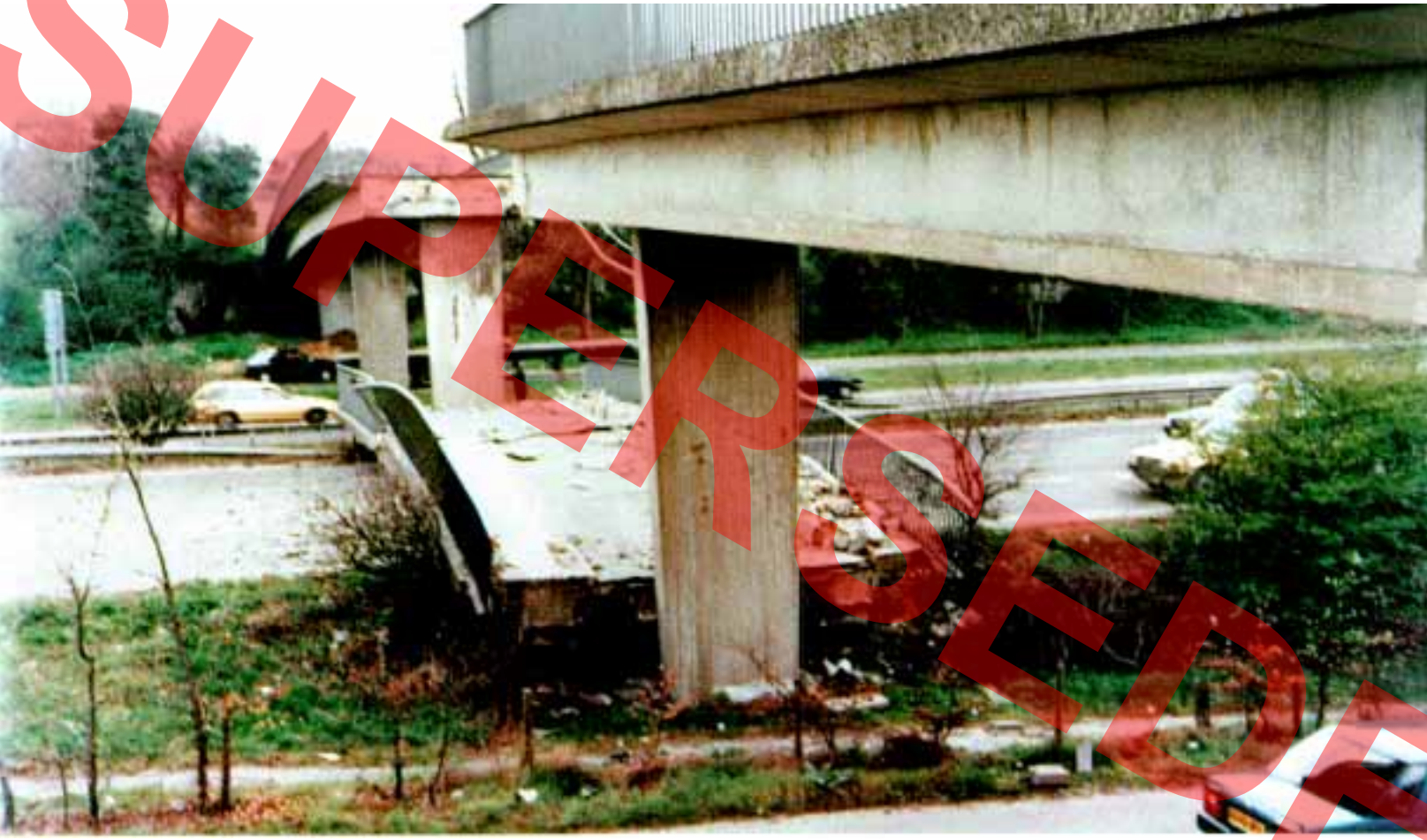
PLATE 2 COLLAPSE OF A DECK SPAN FOLLOWING A COLLISION FROM AN EXCAVATOR TRANSPORTED ON A LOW LOADER A2 PARK PALE ACCOMMODATION BRIDGE
