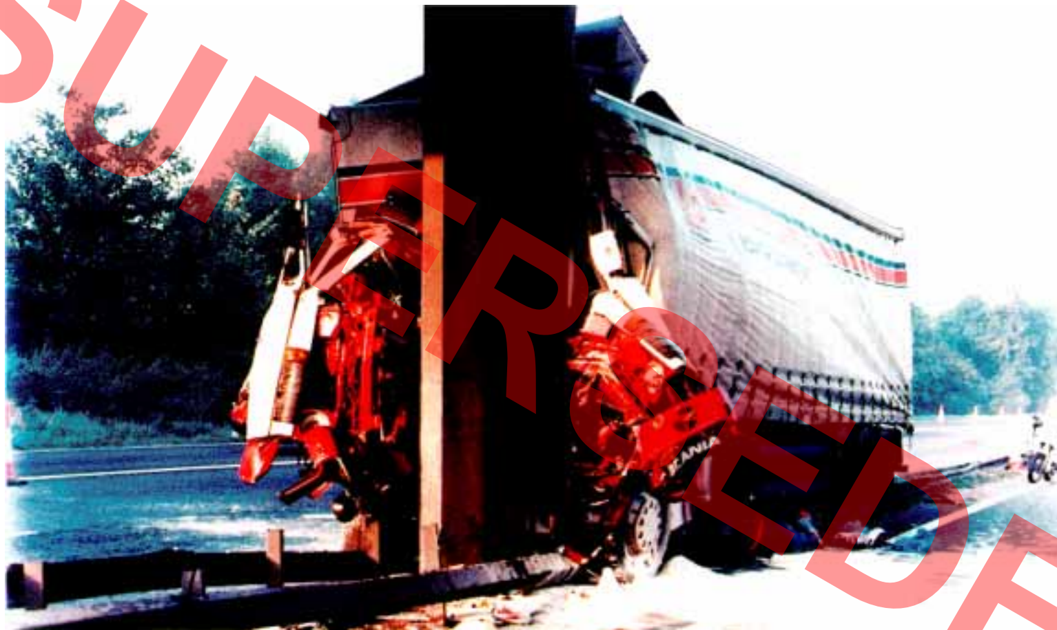
PLATE 1 COLLISION OF HGV WITH REINFORCED CONCRETE SUPPORT M20 BOXLEY ROAD BRIDGE (Photograph by kind permission of Director of Highways and Transportation, Kent County Council)
