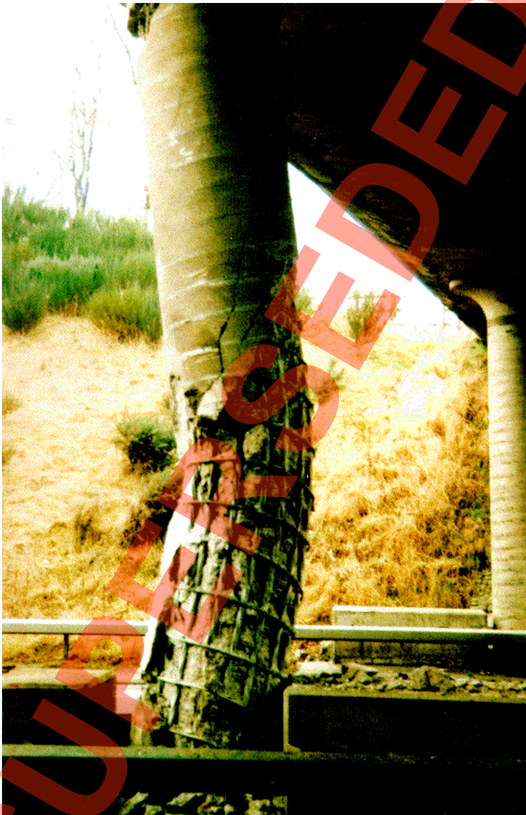
PLATE 3 COLLISION DAMAGE TO REINFORCED CONCRETE CENTRAL SUPPORT M74 LAIRS FLYOVER - B7078
