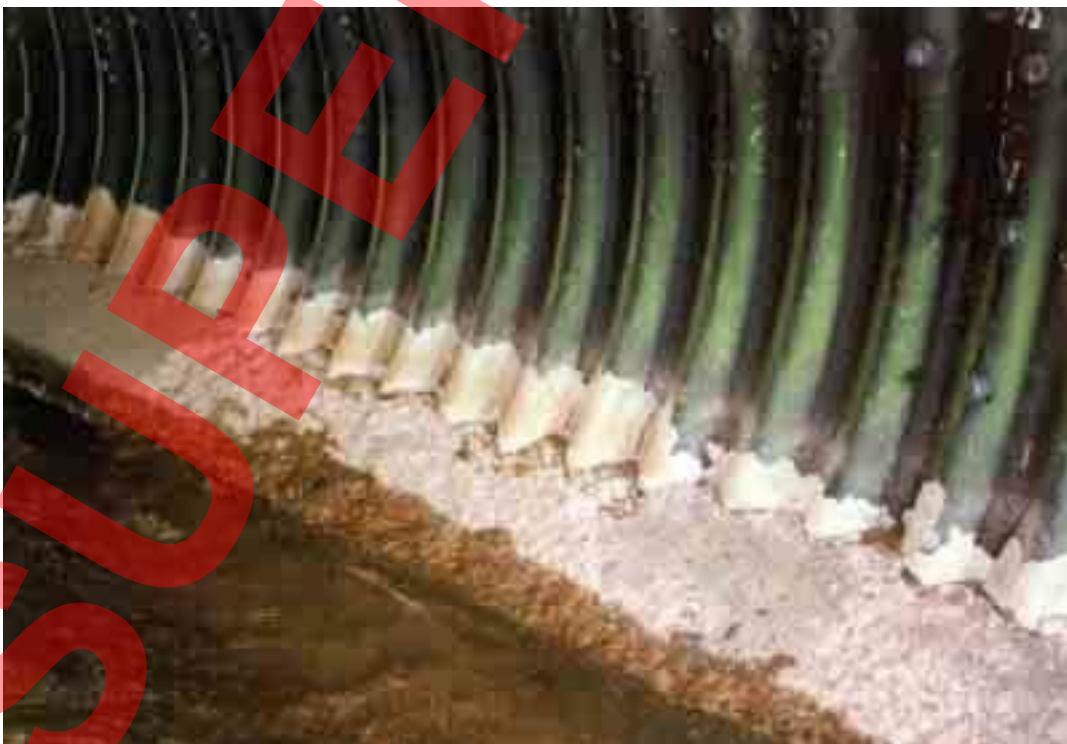
Figure B.3 Damaged bitumen coating caused by overtopping of paving during turbulent flow
