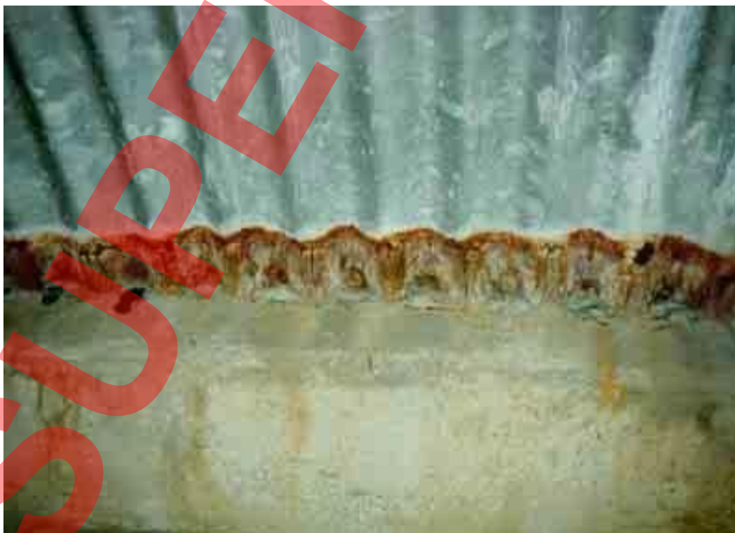
Figure B.9 Deterioration at the arch seating of a plain galvanised arch structure due to seepage and ponding of water containing de-icing salts
