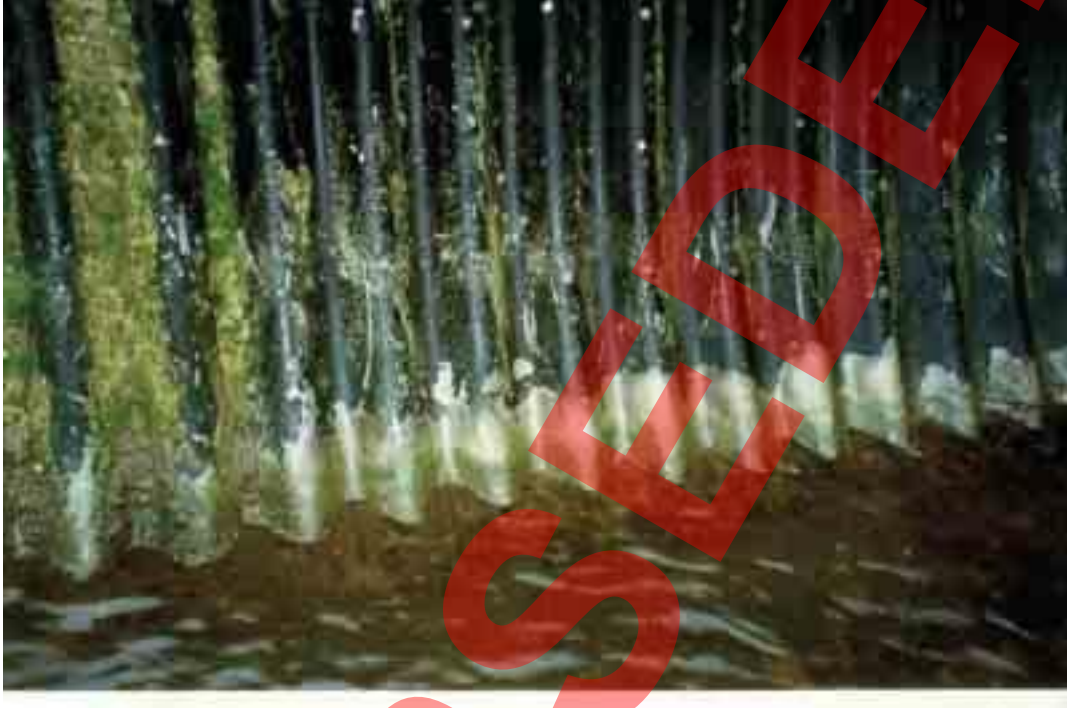
Figure B.2 Deterioration of bitumen coating along the wet/dry line in low flow condition
