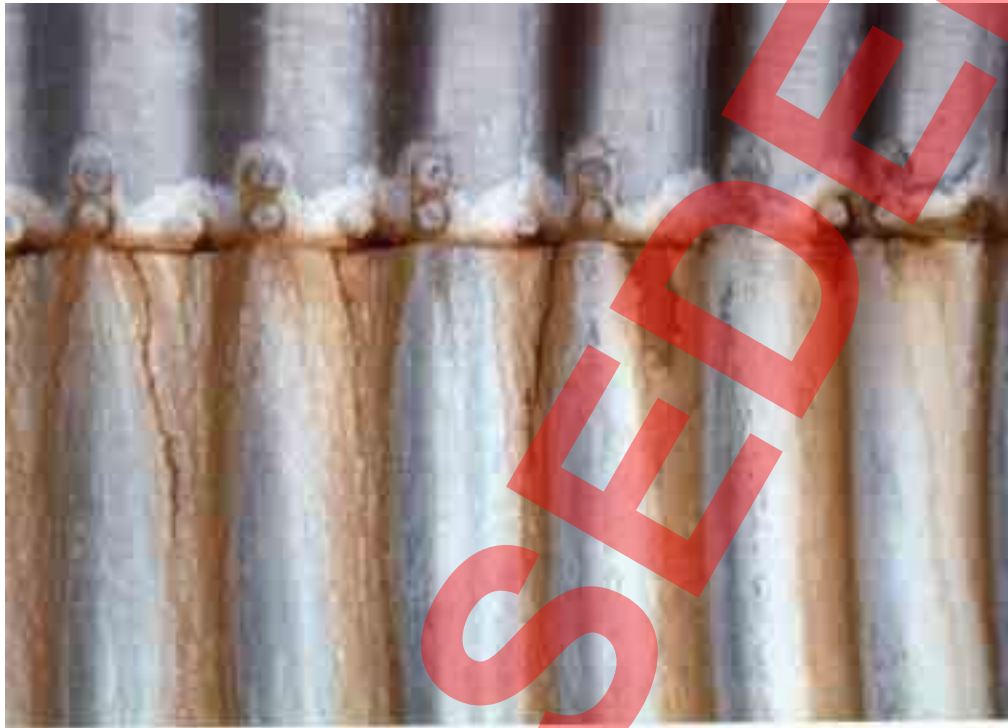
Figure B.8 Deterioration to side plates in a plain galvanised bolted segmental CSBS caused by seepage below the edge of the carriageway
