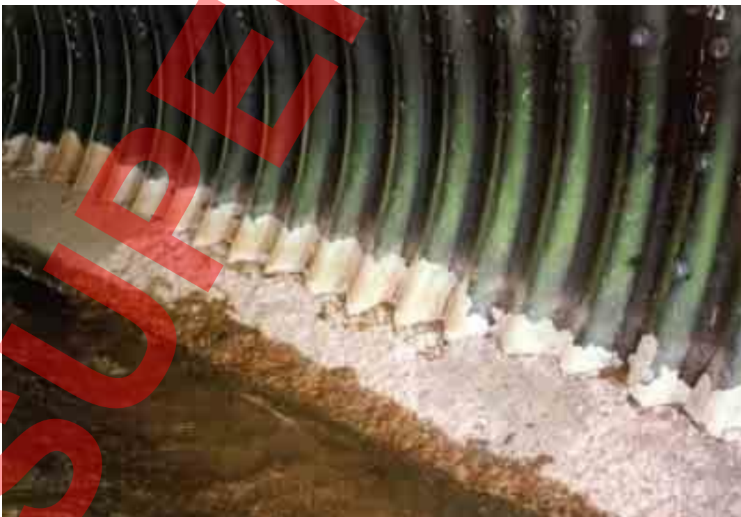
Figure B.3 Damaged bitumen coating caused by overtopping of paving during turbulent flow
