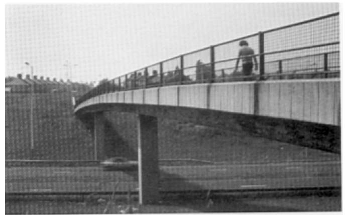
Figure 15. Streaking due to a mistake in detailing. The top of the fascia/parapet plinth was detailed without an inward fall. Correctly detailed bridges with similar parapets on the same contract are not streaked.
