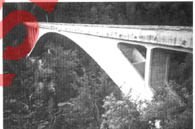
Figure 7. The scuppers in the parapet of the Salginatobel Bridge are there to allow water from the deck to drain away. They also add interest to the bridge when seen close to, and reduce the apparent scale. There may be more scuppers than function strictly requires.
