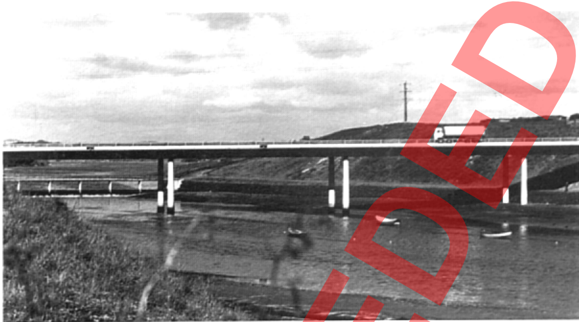
Figure 6. The effect of a light fascia over beams shaded by a substantial cantilever. This is less marked when the sky is overcast.
