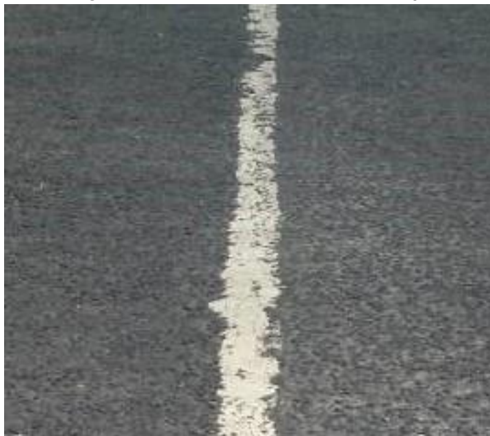
Figure C.8 Condition score 20 – close-up
