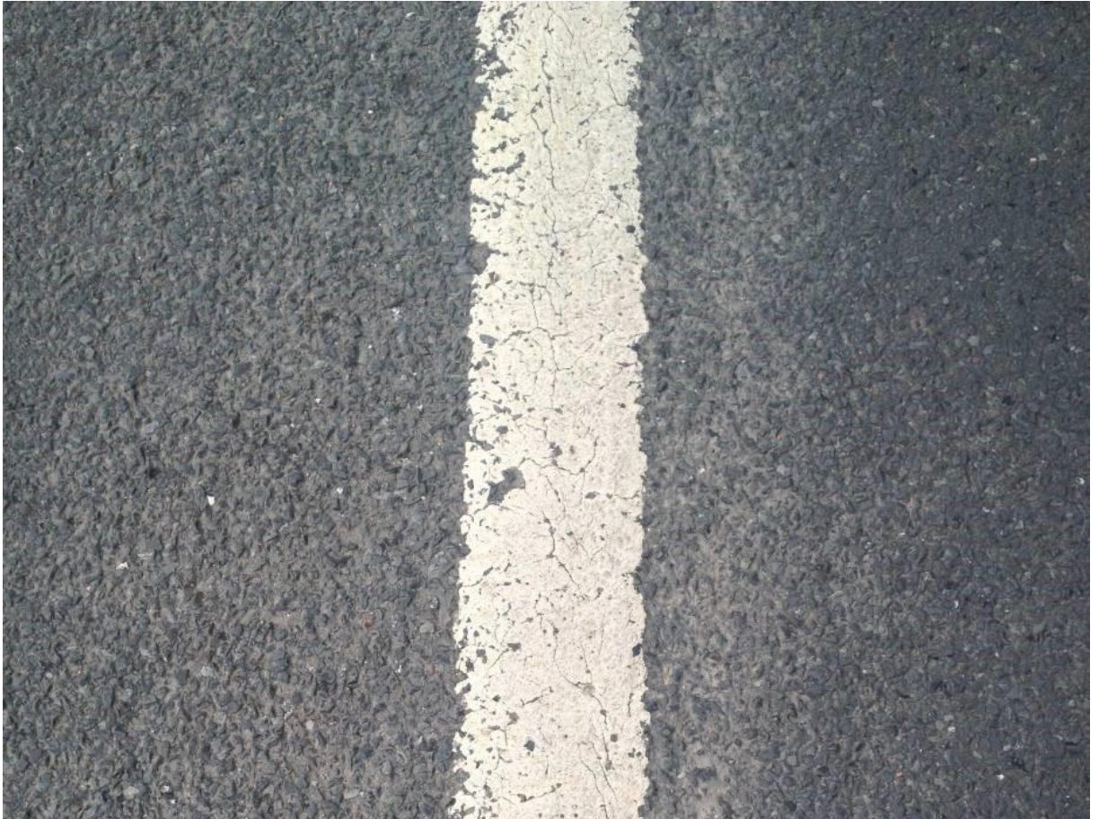
Figure C.6 Condition score 30 – close-up
