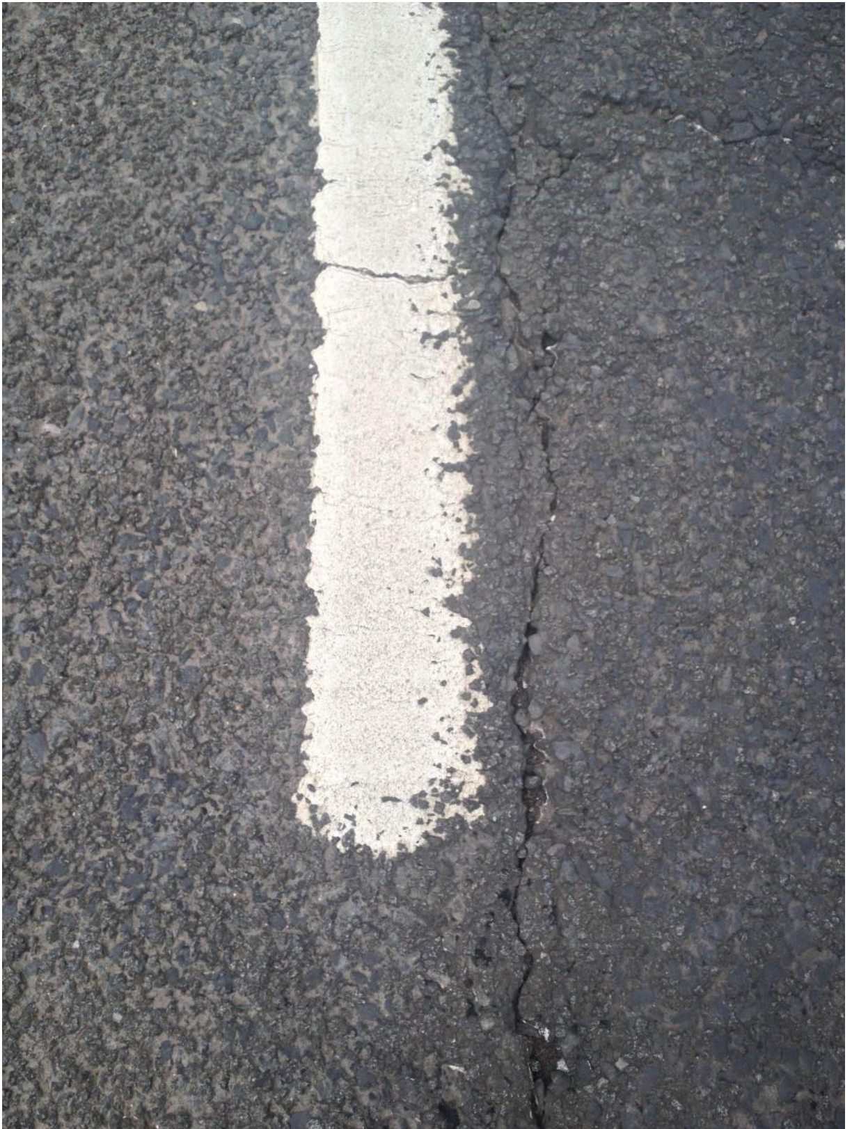
Figure C.4 Condition score 40 - close-up
