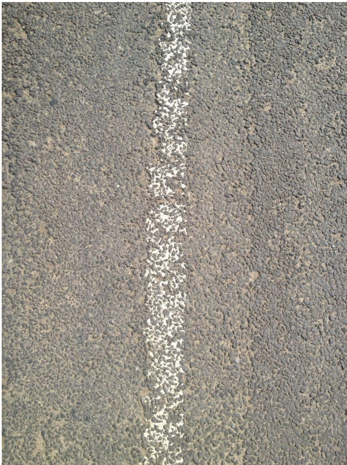
Figure C.11 Condition score 10 – close-up
