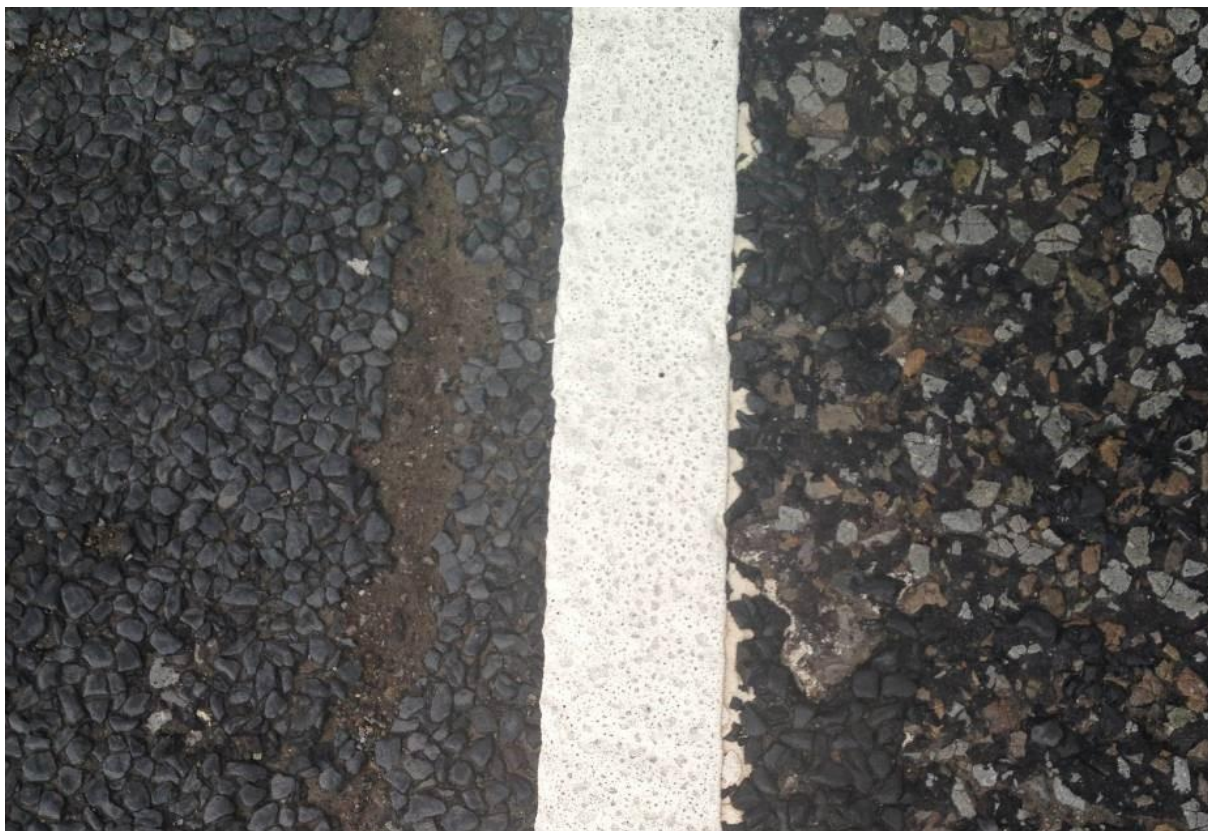
Figure C.1 Condition score 50 – close-up
