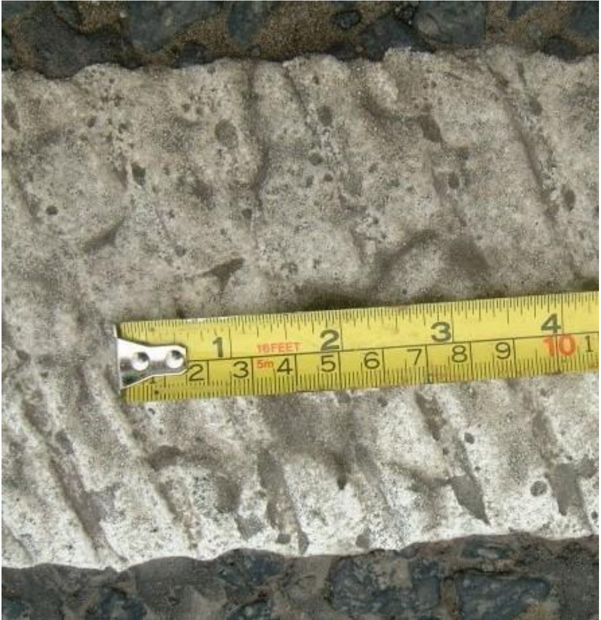
Figure C.9 Condition score 20 – close-up of profiled line designed for wet visibility
