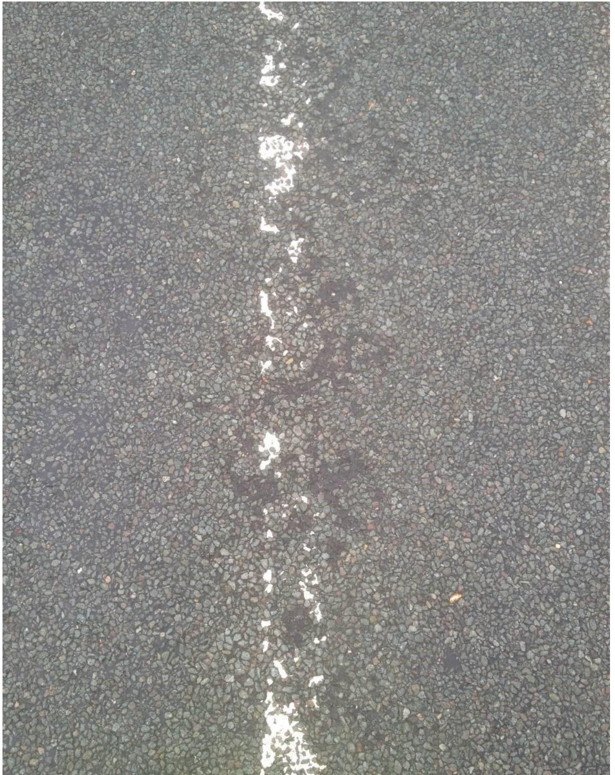
Figure C.13 Condition score 0 – close-up
