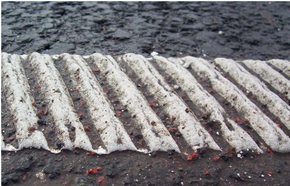
Figure C.2 Condition score 50 – close-up of profiled line designed for wet visibility
