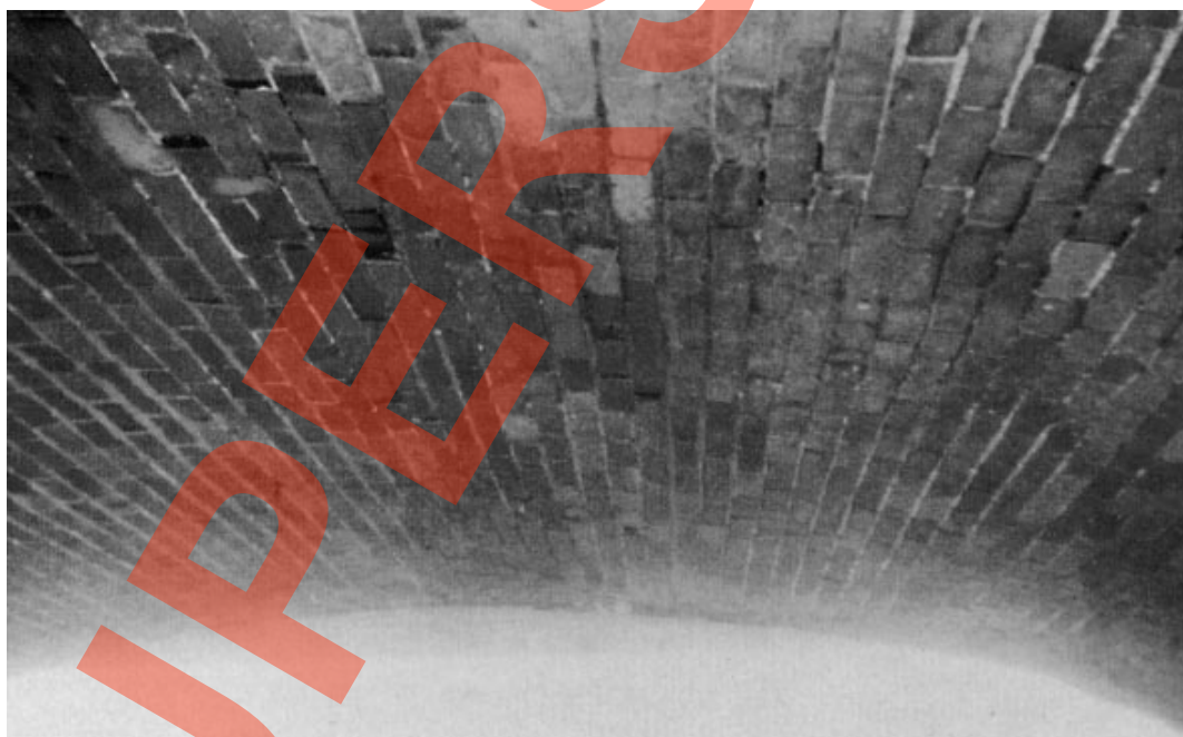
Plate 7 This shows a localised deformation of an arch which would perhaps reduce its Condition Factor by 0.1.
