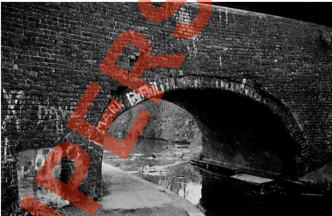
Plate 9 This illustrates the movement of spandrel walls.
