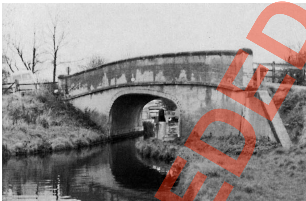
Plate 6 This shows an arch which has become grossly deformed and flattened in shape. The MEXE method would not be suitable for assessing its carrying capacity and instead it should be assessed from first principles.
