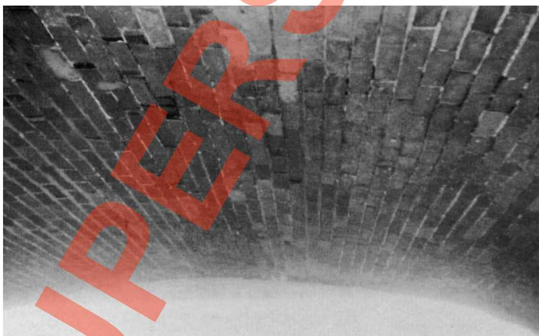
Plate 7 This shows a localised deformation of an arch which would perhaps reduce its Condition Factor by 0.1.
