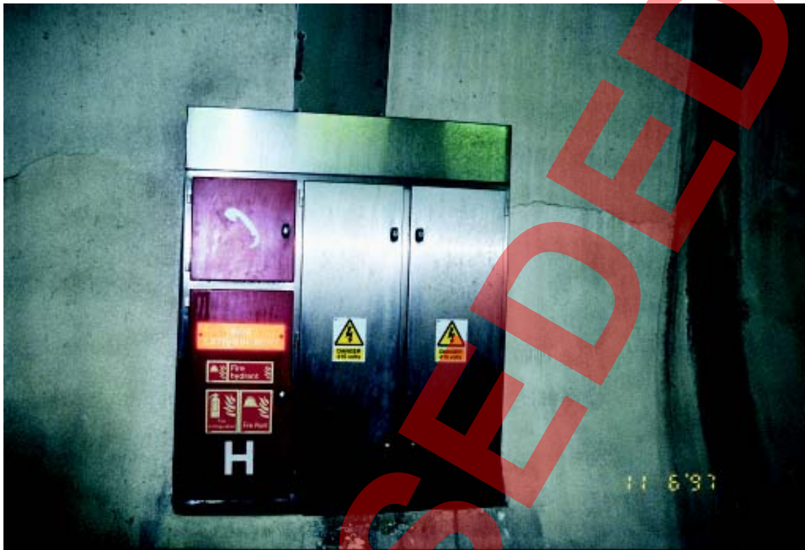
Figure 10.1: Tunnel Emergency Panel
