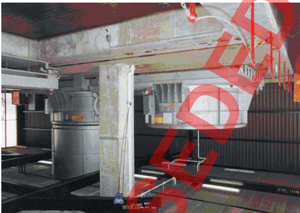
Figure 7.3: Axial Fans on Motorised Duty/Standby Trolley over Supply Shaft
