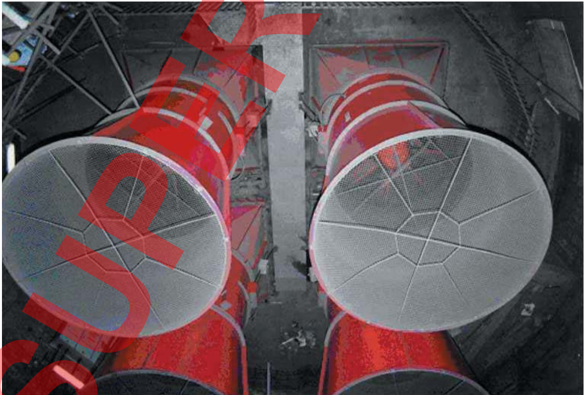
Figure 7.2: Fixed Axial Fans over Supply/Extract Shaft
