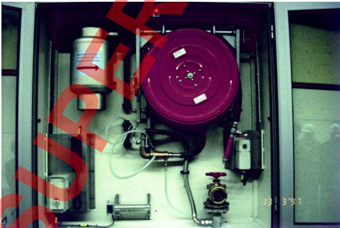
Figure 10.2: Tunnel Fire Fighting Equipment
